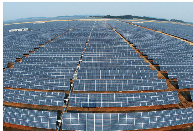
Figure 12. PV power system of 24 MW: SinAn, South Korea of 600,000 m 2 area, [13].
