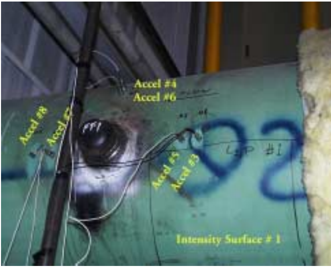
Figure 5. Accelerometer locations and repaired region.
