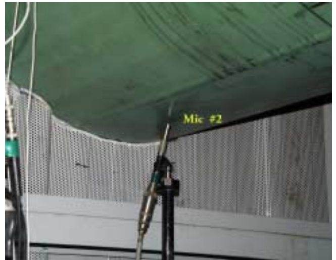
Figure 9. Near field microphone for sound pressure measurement in the discharge piping.
