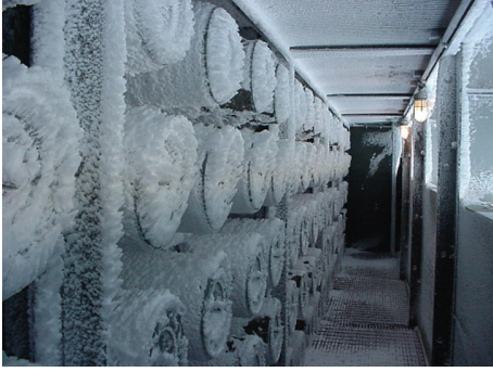
FIGURE 5: Pulse cartridge filters with frost build up due to cooling tower drift [29].
