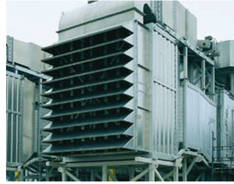
FIGURE 4: Weather Hood on inlet filtration system [34].
