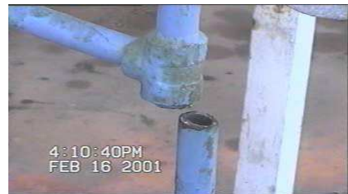
Figure 4. Broken pipeline caused by vibrations
