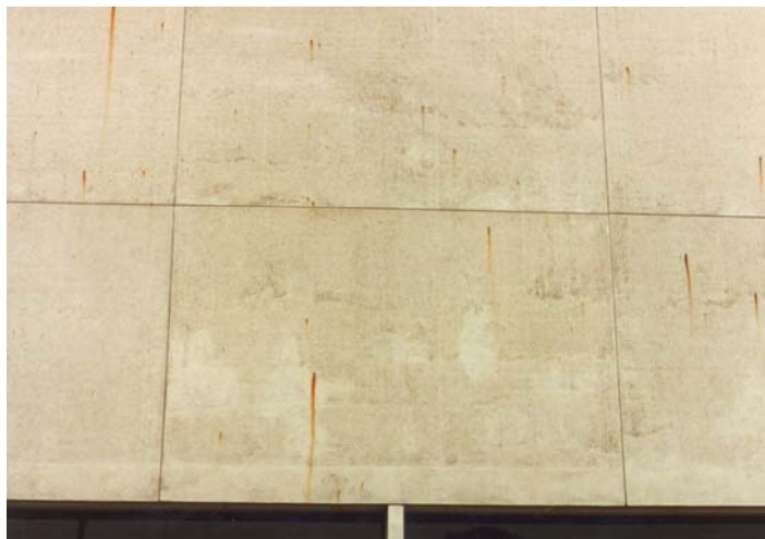
Figure 4. View of pyrite staining on wall panel
