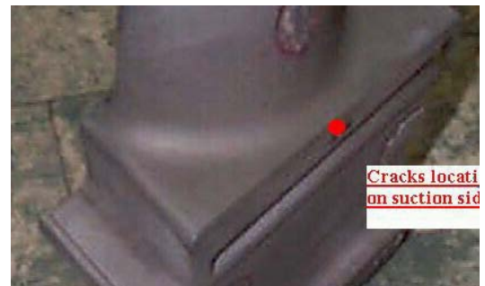
Figure 8 – Position of platform crack shown in Fig. 7.
