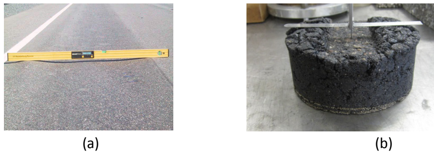
FIGURE 4. Field and laboratory measuring of HMA rutting depth
