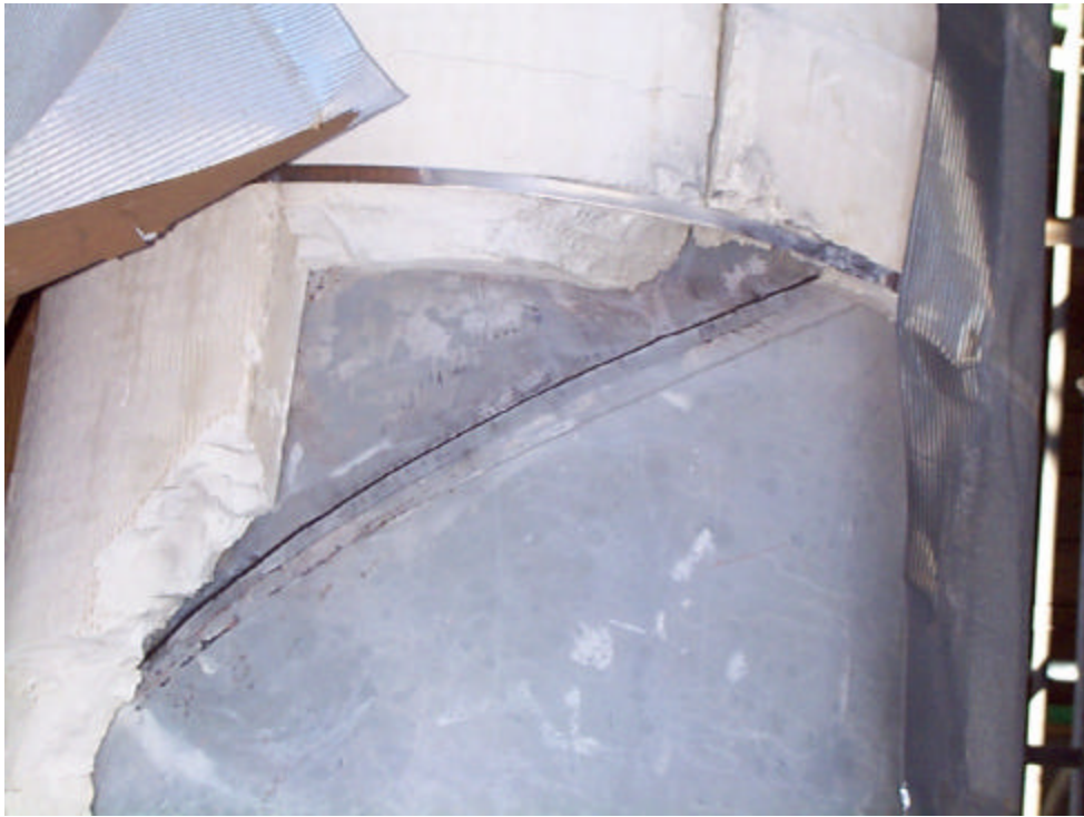
Figure 1: Picture Of Pipe With a Spiral Weld
