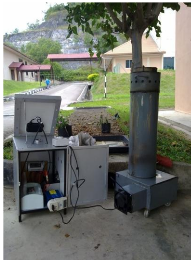
Fig. 2: PV-battery-inverter unit connected to the Belonio rice husk gasifier. PV module tilt angle shown for illustrative purposes only.
