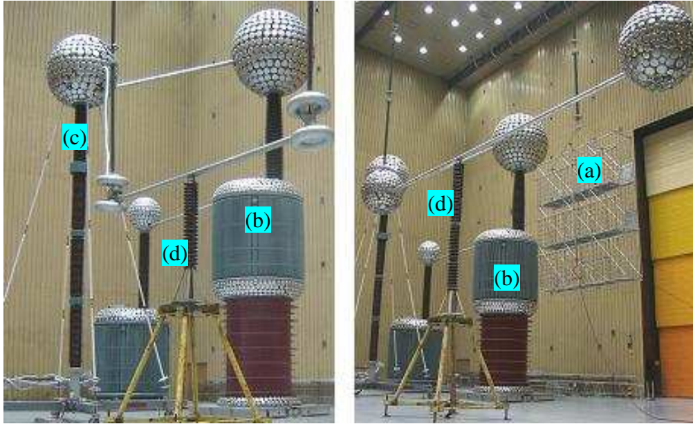
(i) One section under dry test (ii) Full column under wet test (a) artificial rain structure; (b) HV test transformer; (c) voltage divider; (d) insulator under test Figure 2 – Test arrangements
