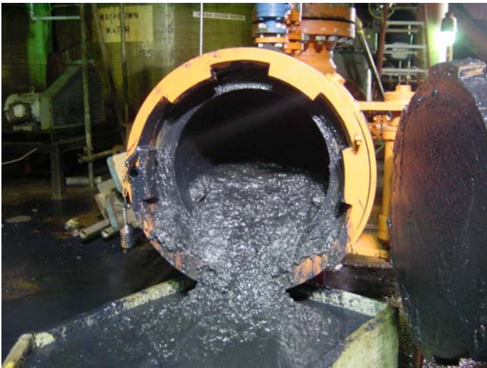
Figure 7 – Receiver on Pouli platform with pigged debris.
