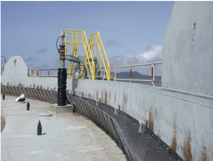
Figure 9 – Secondary floating roof seal on oil storage tank.
