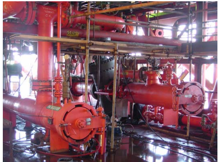
Figure 5 – Two 18” pig traps installed on Poui. Note angled gate valve (grey) on the right trap.
