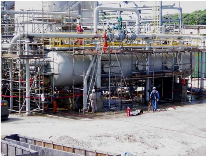
Figure 6 – New separator at the Galeota Point oil terminal to collect pigging debris from incoming pipelines.
