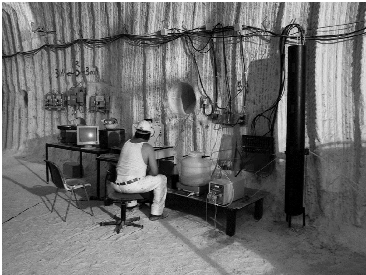
Fig. 13: Preparation of a large borehole (1 m in diameter) in a rocksalt formation in the Asse mine for the emplacement of a SVV seal flooded with a NaCl-rich brine [11]
