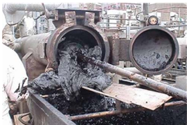
FIGURE 4: FAILURE TO CLEAN PIPELINE ADEQUATELY
