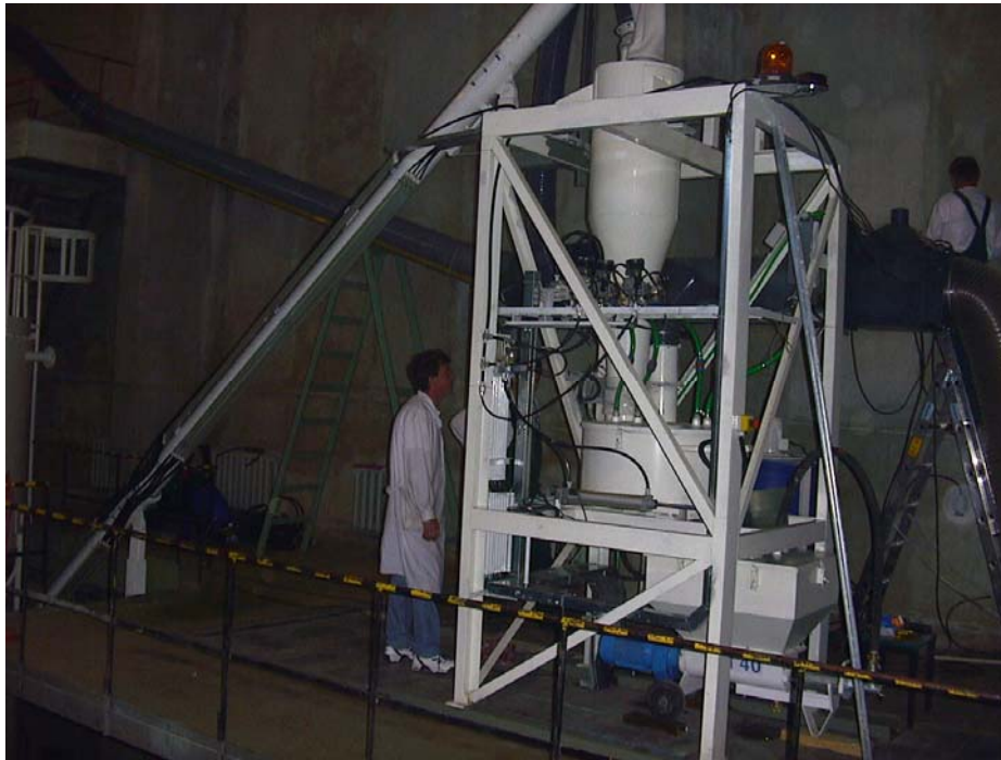
Fig. 2. Salaspils IRT reactor, Latvia, installation of the IAEA-procured cementation plant in preparation to decommissioning
