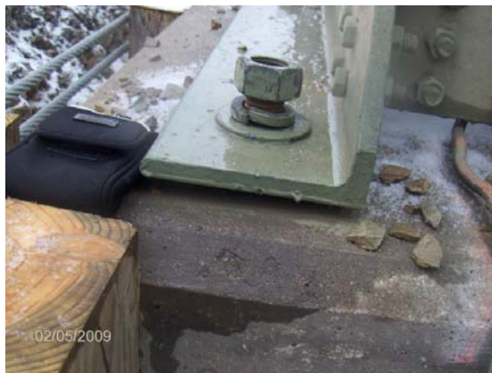
Figure 14. Loosening of the bolts of the connection of the structure to a footing.
