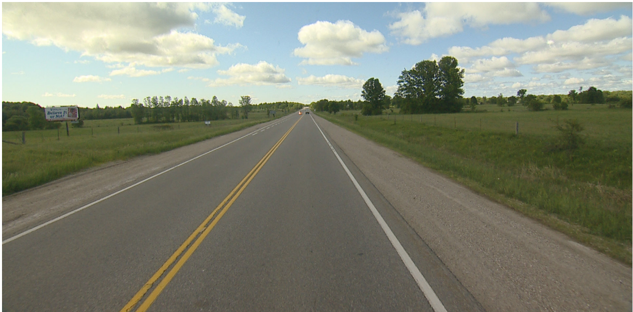
Figure 9. Highway 7 Pavement Condition (2013)
