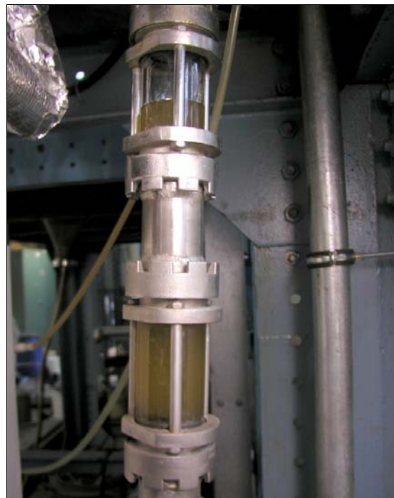
Fig. 1. Sight glass below the condenser with condensate and oil phase
