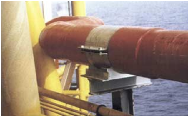
Fig. 2 Pipe on the deck of a TLP
