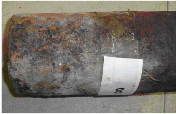
Fig. 4 Corrosion dent of iron casing pipe
