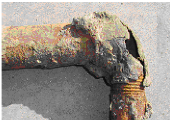
Fig. 5 Corrosion of steel elbow
