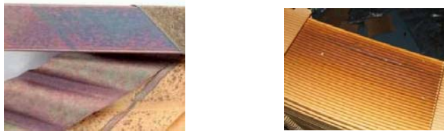
Fig 1. Corroded copper conductor (left) showing clear \text{Cu}_2\text{S} deposition on the wrapping paper. Right shows deposits on paper between spacers in disc winding. This type often also contains sludge.
