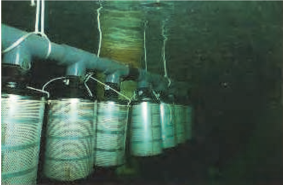
Fig. 4. UCC vacuuming filtration system underwater manifold.
