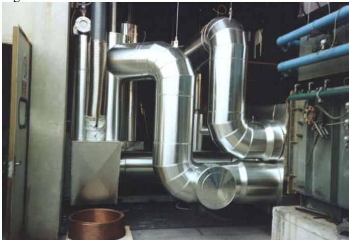
Figure 2 - Front view of the microturbine recuperator (bottom left of the picture), which has been displaced from its original position within the package (courtesy of ARI)
