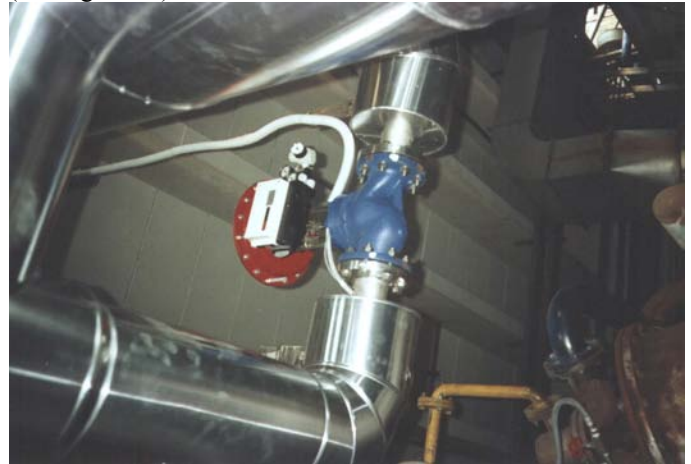
Figure 3 - View of the bypass valve V_A (courtesy of ARI)
