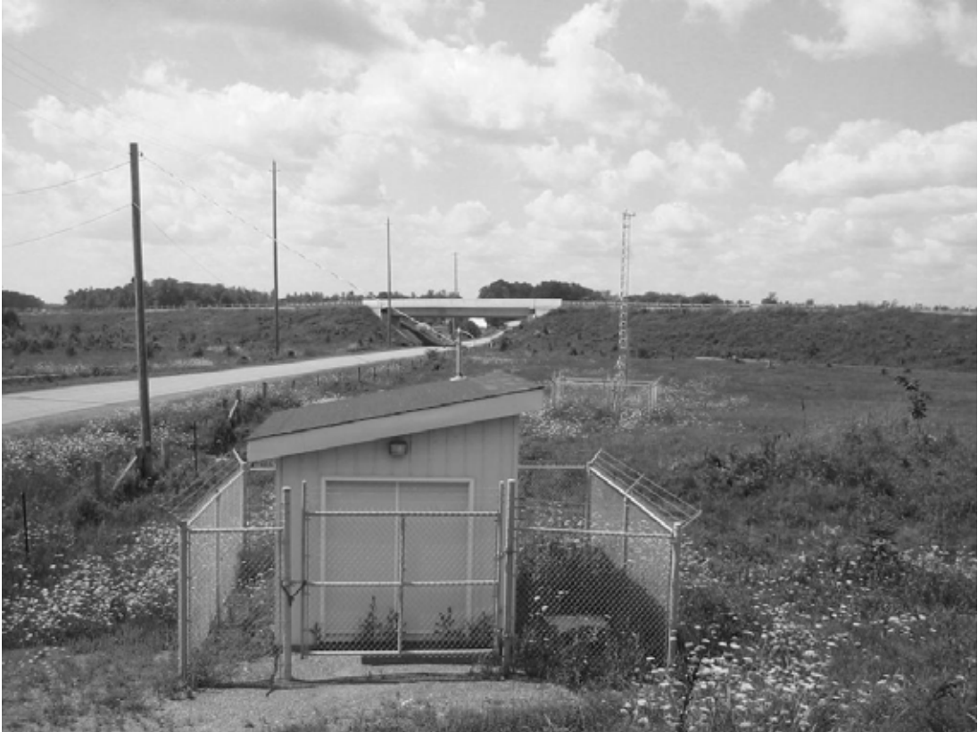
Photo courtesy of Boschung America, LLC
