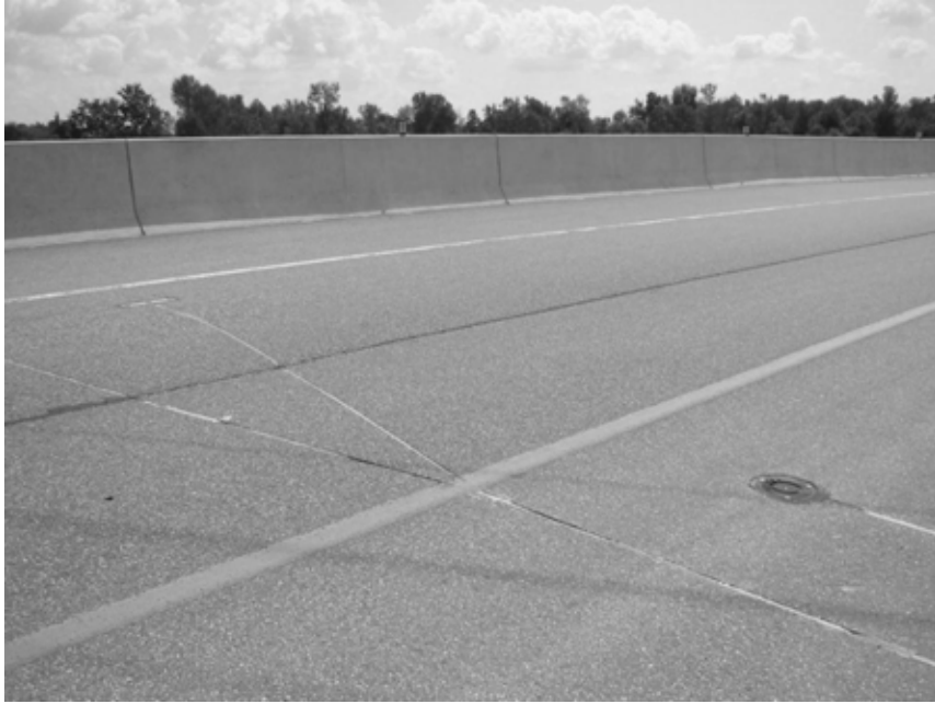
Photo Courtesy of Boschung America, LLC
