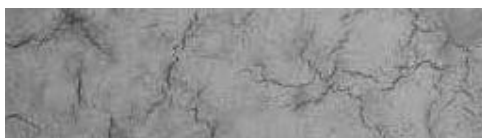
Figure 3 Removal of Cracks from the Gray Scaled Image
