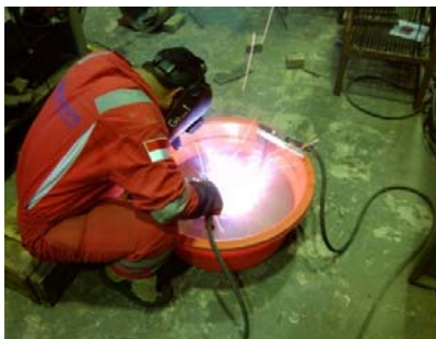
Figure-4. Underwater wet welding process in the plastic tub containing the artificial sea water.
