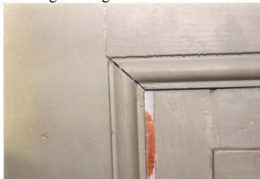
Figure 4. One of the panels hanging loose in the frame
