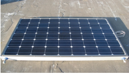
FIGURE 4: Unglazed PVT collector.
