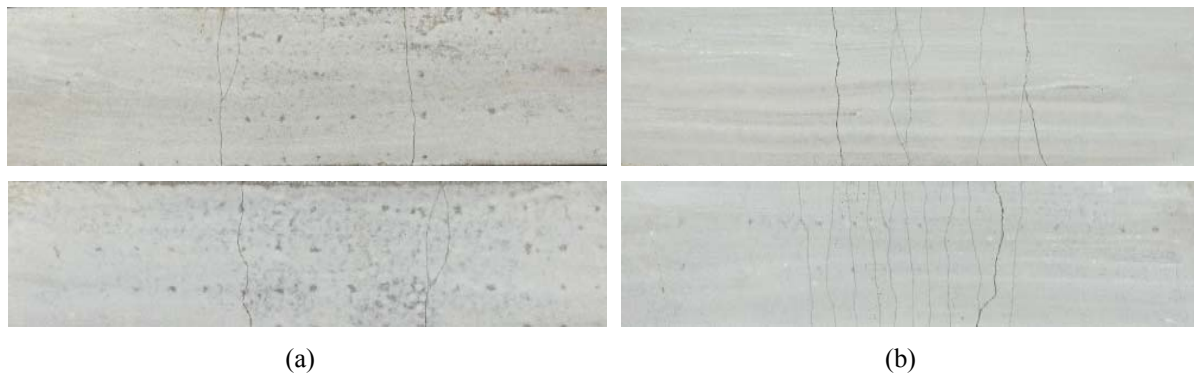
Figure 6: Typical cracking patterns For: (a) R2%_50 composite and (b) R4%_50 composite.
