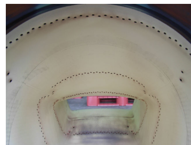
Figure 10. Picture of combustion liner at inspection (Verification operating time 681 hour/51 start and stop)
