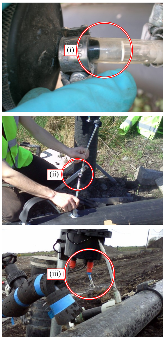
Figure 4: Site-specific issue rectification (i) Water blockage, (ii) Tube shrinkage, (iii) Connection breakage due to pipe collapse
