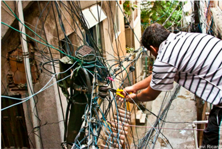
Figure 1. A confusion of overhead cables in Favela da Rocinha. Photo credit: Levi Ricardo.
