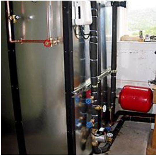
Fig. 3 A portion of the plumbing system
