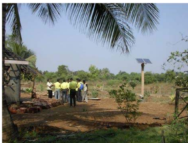
Fig 7 Cottage industry group in India installing a pole mount PV system at a “green” resort near Mumbai.
