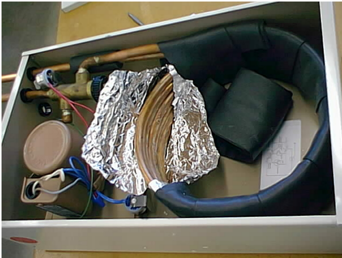
FIGURE 3. HEAT CONTROLLER DS06, COILS EXPOSED.
