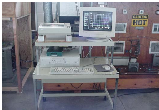
FIGURE 9. DATA ACQUISITION SYSTEM CONNECTED TO NEWLY INSTALLED HEAT PUMP.
