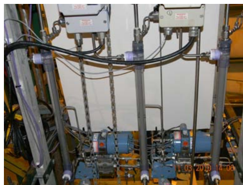
FIGURE 5. THREE FILTER TUBES IN FILTER HOUSINGS
