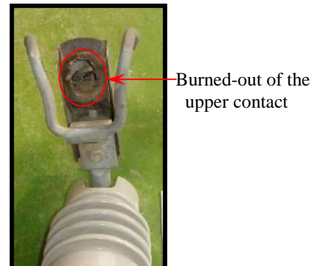
Fig. 2: Burned-out of the upper stationary contact on PRW type drop-out fuse
