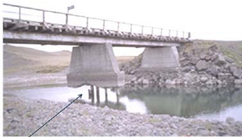
Scour Fig.2 Bridge scour [1]
