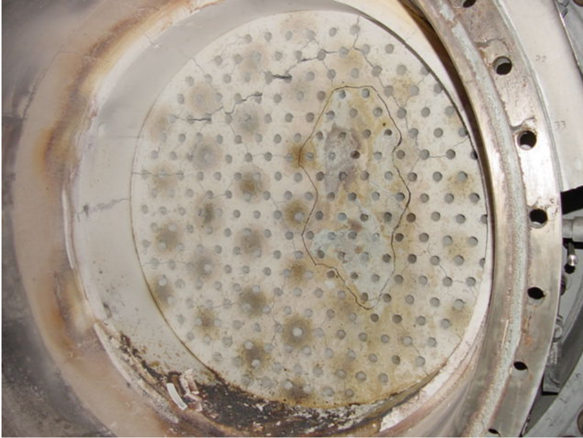
Figure 3 Picture of failed pulse combustor tube sheet.
