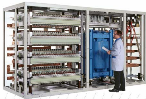
Fig.3: One-half of a 65 Megawatt LCI-type frequency converter or „drive“ for the motor shown in Fig. 1.
