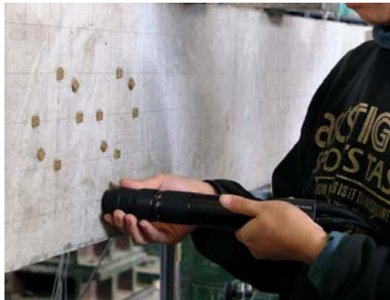
Fig. 3 Measuring crack width by using digital microscope
