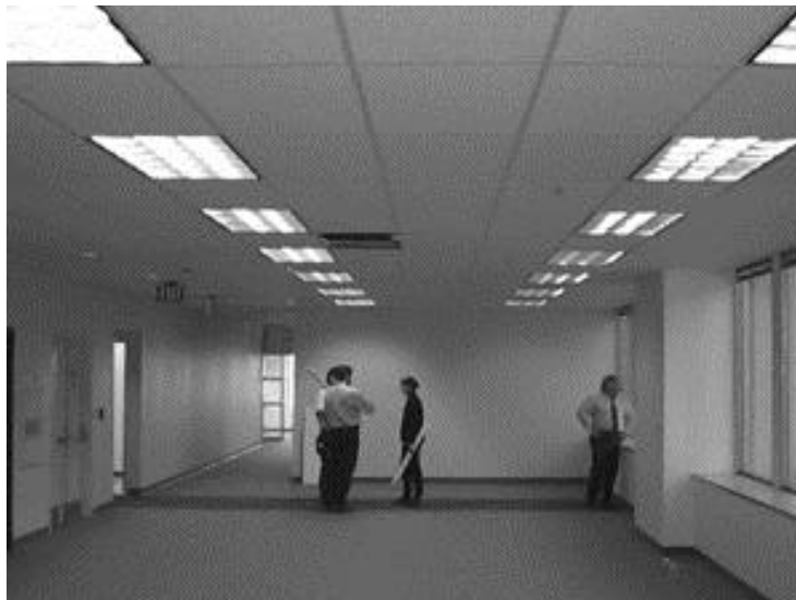
Figure 2. An interior view of the third floor taken during commissioning of the lighting system before installation of the furniture system. Note the luminance pattern on the far wall which shows that the row of lights nearest the window is heavily dimmed while the second row is at near full intensity.
