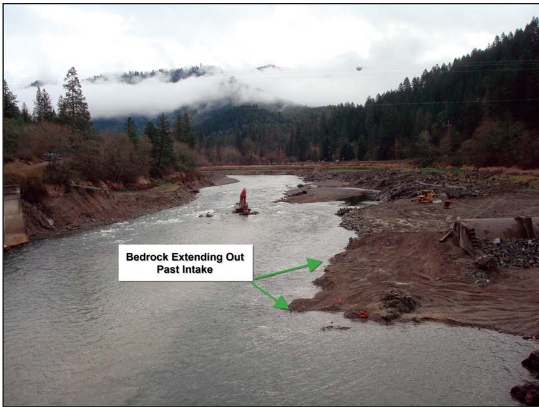
Figure 10. Looking upstream near the end of the February 2010 excavation work, noting bedrock that extended farther out than estimated.
