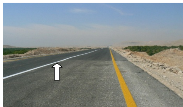
Figure 3. A heave in asphalt layer of the studied road due to swelling of the expansive soil sub-grade at El-Kawther sector.
