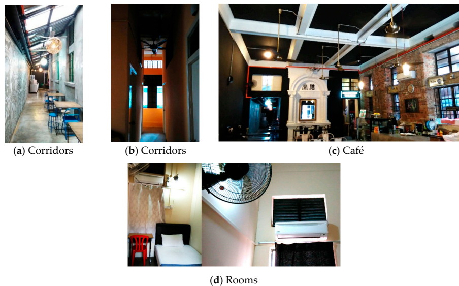
Figure 6. Types of mechanical ventilation in corridors, café and rooms in Building A.
