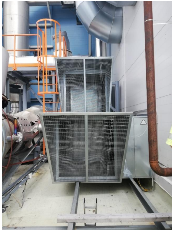
Figure 9. Test cell air ventilation outlet on the laboratory roof.
