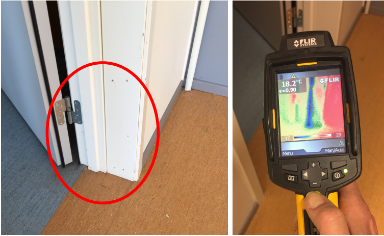
Figure 5.7: To the left is a photograph and to the right is a thermography of air leakage location L4. The air is leaking through cracks in the connection of the door frame to the inner wall and floor.
