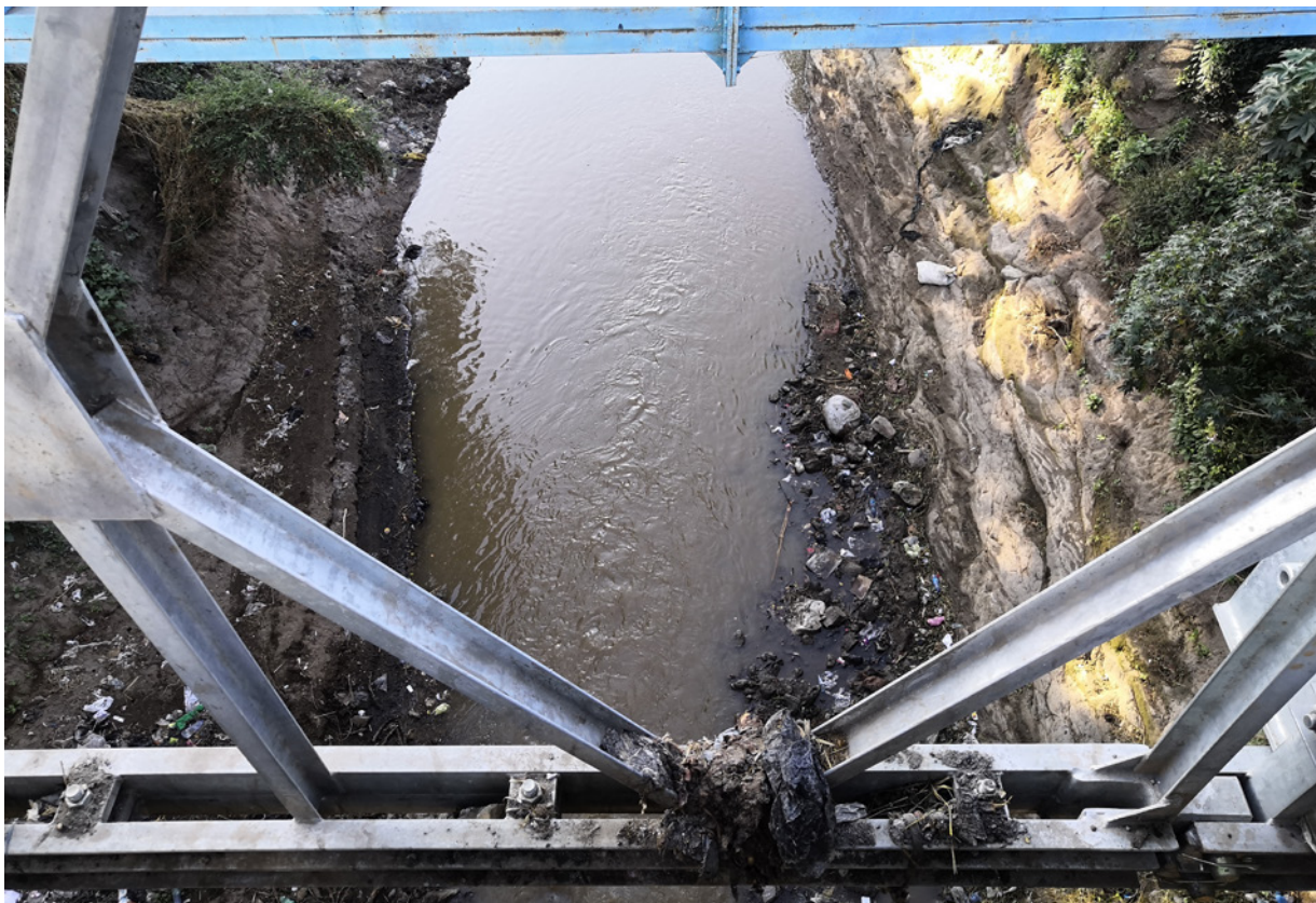
Figure A5.1. The bridge in Meki Town serves as a waste dump. The site is unsafe, dirty and prone to vandalism.
