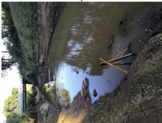
Meki at Meki Town (1): Staff gauge is rusty and the reading has almost disappeared. There are waste and sediment deposits on the riverbanks. Open defecation near the station interferes with data recording.
