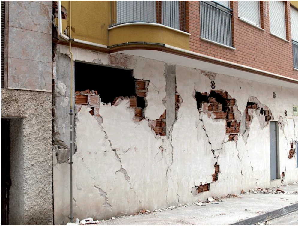
Figure 28. Lorca, X-shaped cracks in infill walls and loss of concrete in the middle body of the RC column suggest a soft story effect. Source: IERD.
