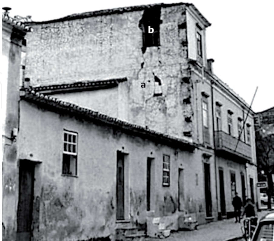
Figure 1. Silves, building of class B with damage of grade 3: (a) shear cracks with detachment of little pieces of plaster; (b) partial toppling of external wall. Source: IPMA.
