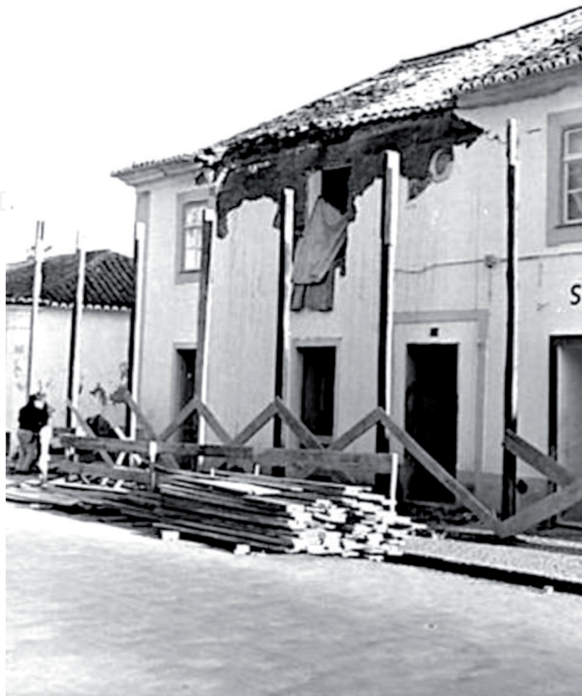
Figure 9. Portimão, two-story building of class B with detachment and toppling of the outer leaf of the external wall on the second floor, due to a hammering effect between the wooden joists supporting the roof and the top of the load-bearing walls (grade 3). The lack of shear cracks indicates a ground displacement from back to front. Source: IPMA.
