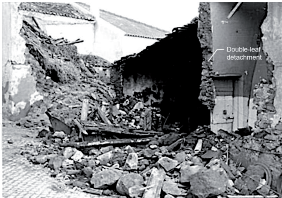
Figure 4. Vila do Bispo, total collapse of building of class A made of mixed fieldstone and adobe masonry, mud or clay mortar and roof supported by wooden logs and bed of reeds (grade 5). See the double-leaf shape on an interior load-bearing wall remaining standing. Source: IPMA.
