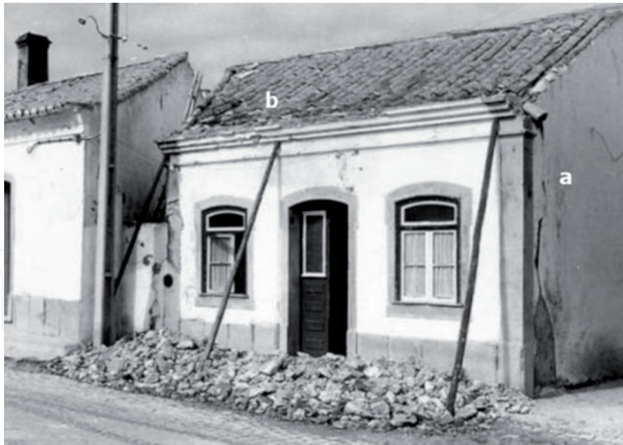
Figure 8. Sagres, building of class A with damage of grade 3: (a) loss of connection of load-bearing walls with drift of façade, and (b) detachment of cornices and tiles with partial roof collapse. Source: IPMA.
