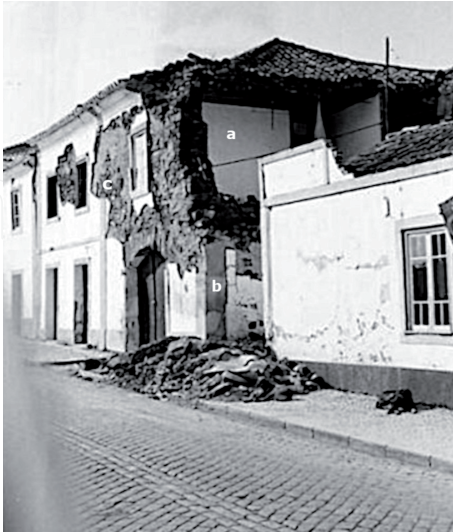
Figure 2. Bensafrim, building of class A with damage of grade 4: (a) advanced corner failure and toppling of external wall with partial roof collapse; (b) loss of connection and drift between load-bearing walls; (c) generalized detachment of plaster. Source: IPMA.
