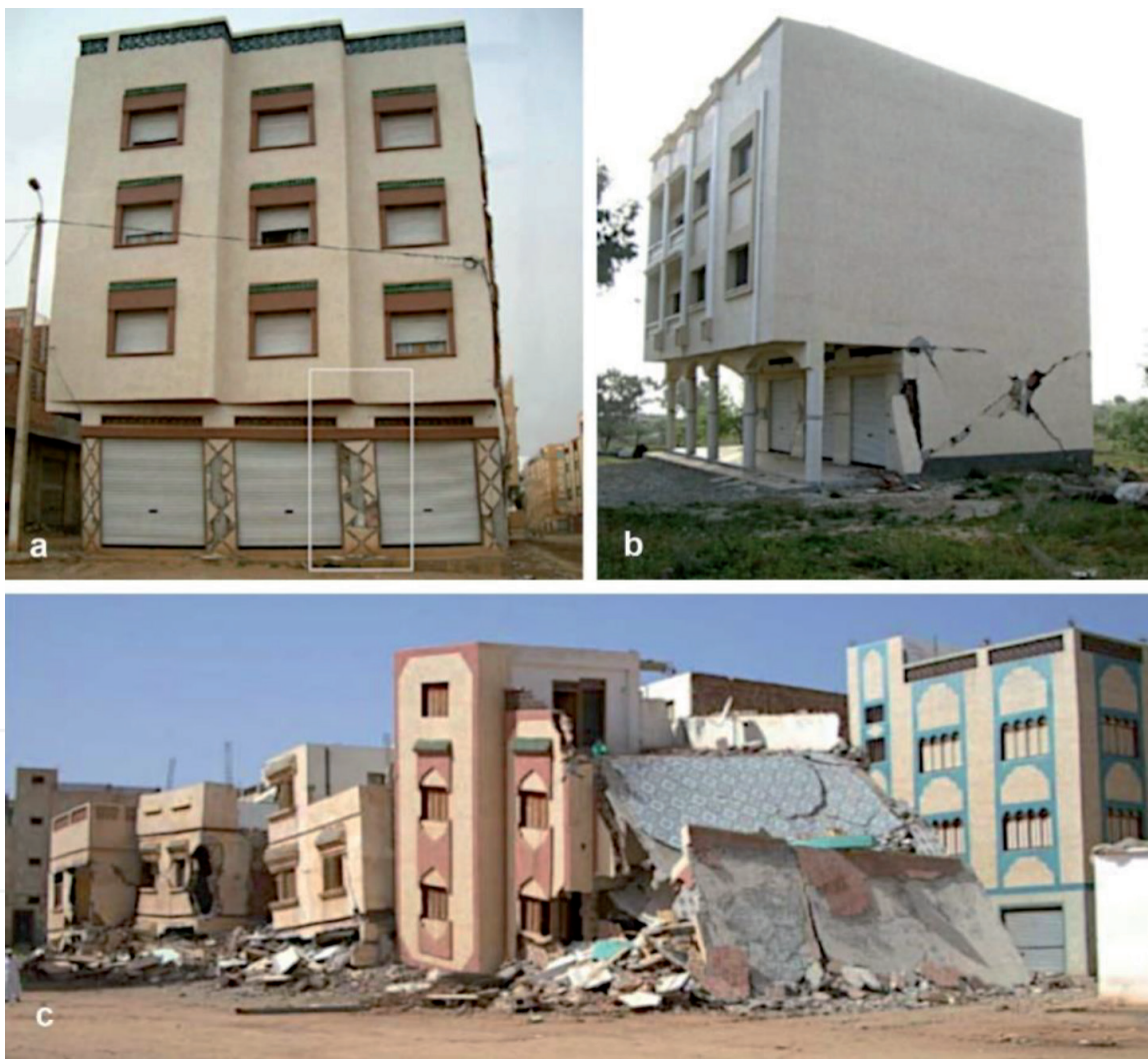
Figure 19. Alhucemas, soft-story failures: (a) tilting of RC frames on the ground floor; (b) soft-story damage with clear X-shaped crack on the infill wall; (c) collapse of ground floor due to a previous soft-story damage. Source: P Murphy.
