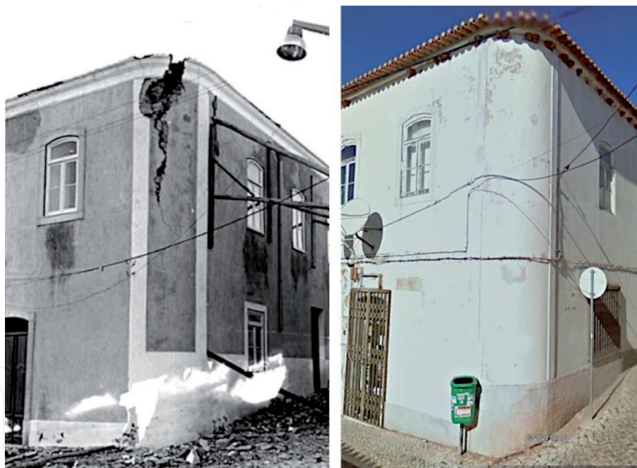
Figure 5. Vila do Bispo, building of class A with damage of grade 3 due to loss of connection between load-bearing walls and corner failure (left). This two-story house was repaired and is currently in use (right). Sources: IPMA/Google Earth.
