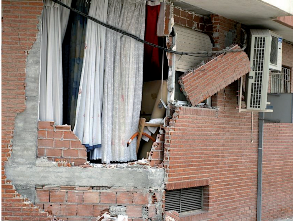
Figure 26. Lorca, complete overturning of double-leaf wall with overturning of both brickwork faces, but without apparent cracks in the RC frame. Source: IERD.
