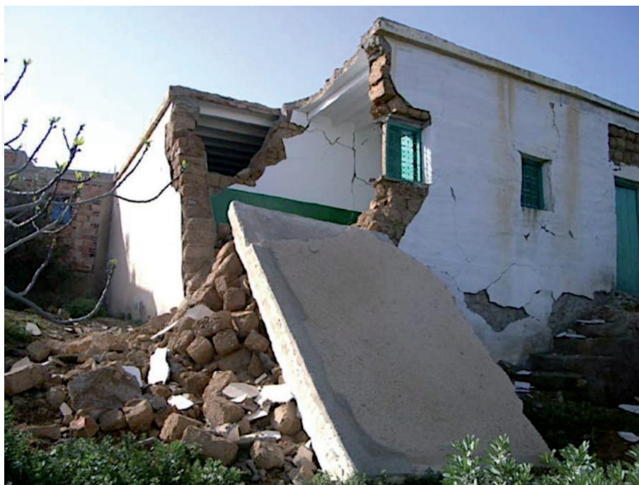
Figure 14. Ait Kamara, corner failure pulling down the roof slab (grade 4, class A). Source: P Murphy.
