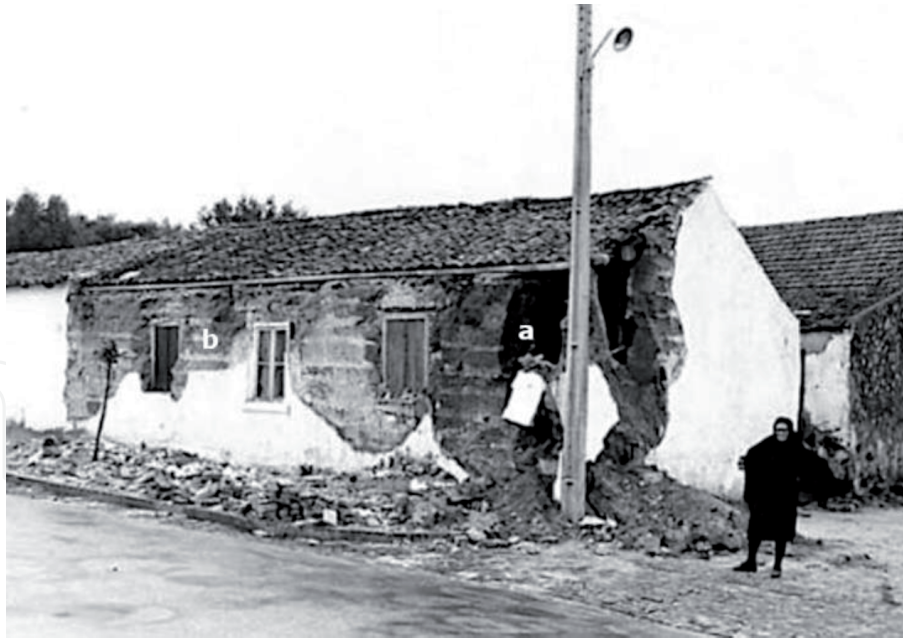
Figure 12. Grândola, damage of grade 4 in a house of class A (adobe masonry): (a) advanced corner failure not compromising the roof; (b) general detachment of plaster. Source: IPMA.
