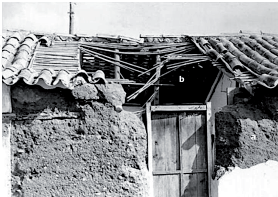
Figure 11. Odemira, damage of grade 4 in adobe masonry house of vulnerability class A: (a) detachment of plaster; (b) partial roof collapse due to the strong pounding of wooden logs against the top of the load-bearing wall. Source: IPMA.
