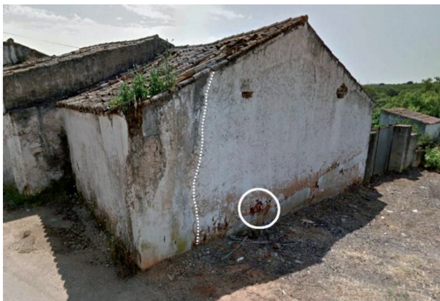
Figure 10. Fonte de Louzeiros, building of class A rebuilt after the 1969 earthquake, showing the repair mark of a corner failure (dotted line). Inside the white circle is visible the red color of the clay used to join the adobe masonry. Source: Google Earth.
