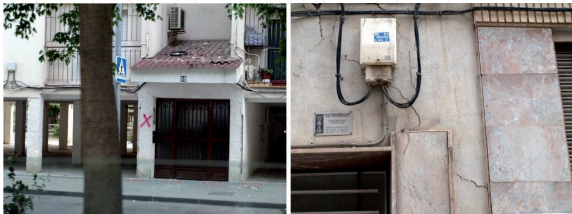
Figure 20. Lorca, shear cracks in pre-1968 RC buildings of class C (grade 3). There is apparently no evidence of structural damage, and on the ground floor (left) the columns forming an evident soft story have no sign of tilting. Source: IERD.
