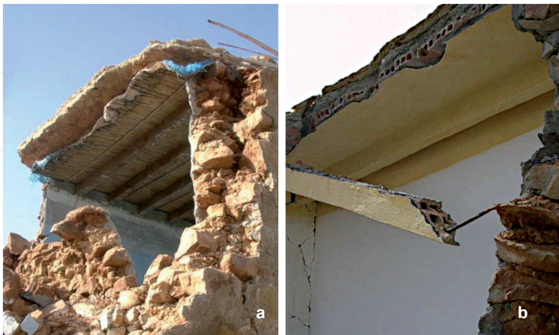
Figure 13. Ait Kamra, traditional house pattern: (a) partial collapse showing the doble-leaf load-bearing walls, fieldstone masonry bonded with mud mortar and roof of wooden logs and canes covered with a plastic film (blue) and layer of water-repellent mortar (grade 4, class A); (b) handmade joist of hollow bricks assembled with a single steel rod. Source: P Murphy.
