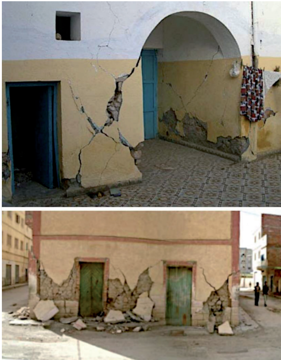
Figure 17. Examples of X-shaped damage clearly visible in a single-story class A house (above) and blurred by loss of outer leaf in a four-story residential block (below). Source: P Murphy.
