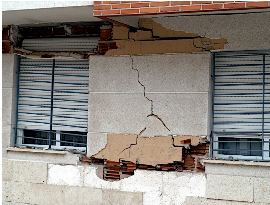
Figure 24. Lorca, loss of stone cladding, fall of window lintel and X-shaped crack on external wall about to fall down. Source: IERD.
