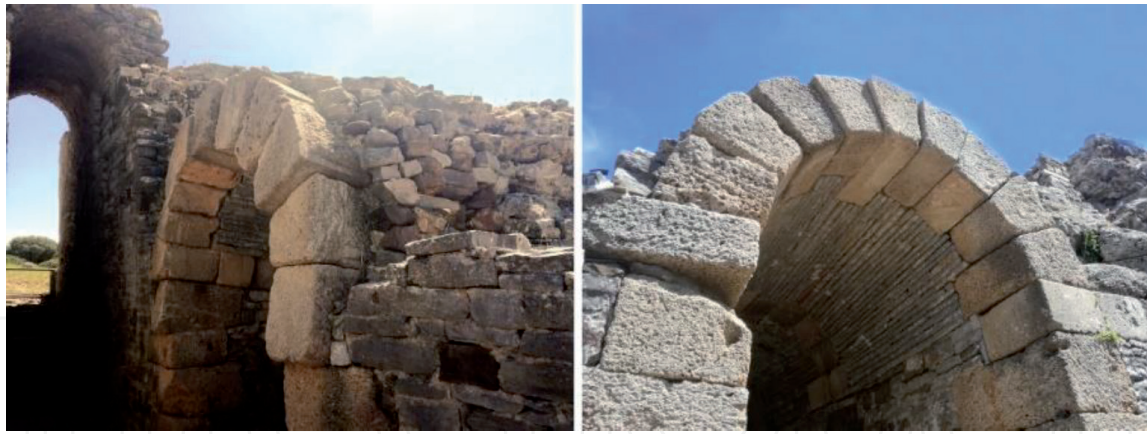
Figure 15. Baelo Claudia, roman ruins (theatre): bowing of a vomitorium wall (left) and expulsion of voussoirs near the parascenium (right), which show a tensile stress in the direction of the slope. Source: J A Aparicio.
