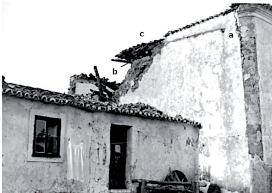
Figure 6. Vila do Bispo, building of class A with damage of grade 4: (a) loss of connection between load-bearing walls; (b) toppling of external wall; (c) collapse of roof made of wooden logs and bed of reeds. Source: IPMA.
