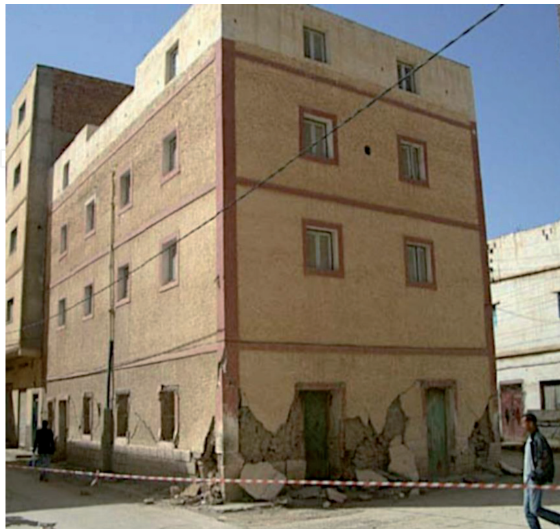
Figure 16. Imzourem, X-shaped damage completely surrounding the load-bearing walls on the ground floor of a four-story residential building of vulnerability class B (grade 3). Source: P Murphy.
