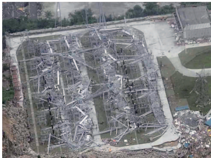
Figure 4. Damage to equipment in the Ertaishan switchyard.
