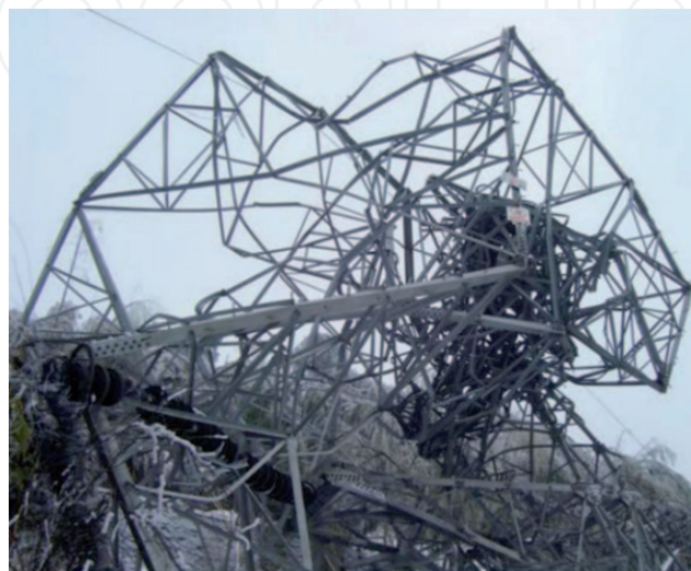
Figure 3. Transmission tower collapse caused by ice accumulation.
