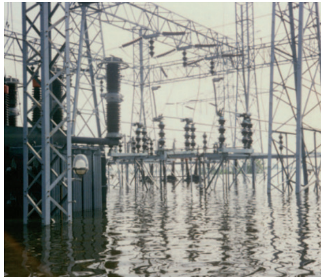
Figure 1. Flooded substations during the 1993 flood at UE.
