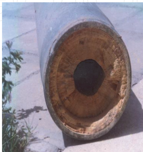
Figure 1. Scaling through \text{CaCO}_3 precipitation in drinking water pipes.
